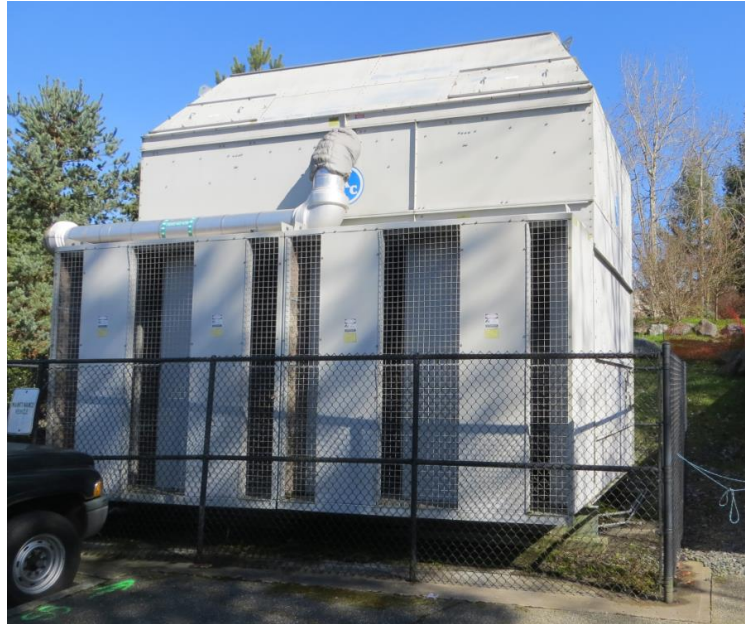
Cooling Tower CT-1
