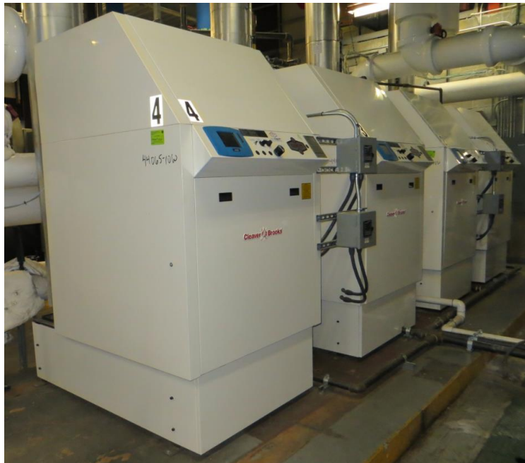
Boilers B-1, B-2, B-3, and B-4
